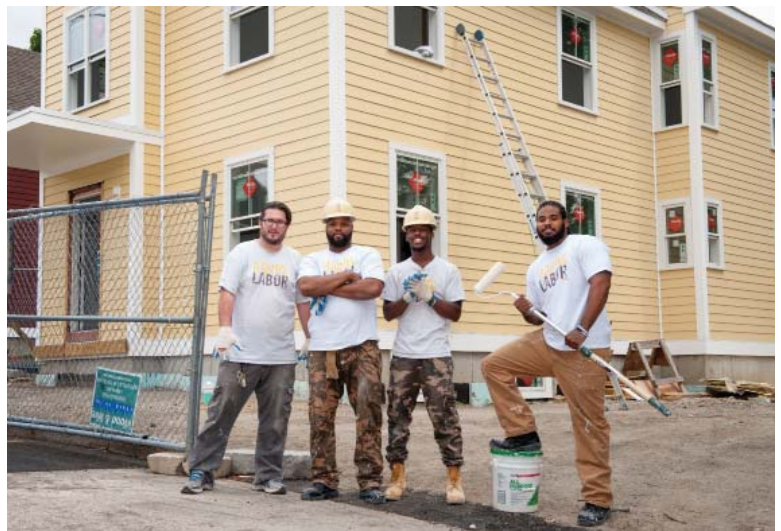
Building affordable housing in Providence as part of a pre-apprenticeship program for the construction trade.
